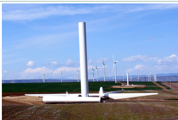
PGE's Biglow Canyon Wind Farm in Sherman County, Oregon. CREDIT: Tedder (2009)
